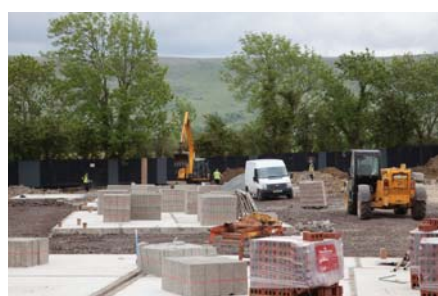
Social housing at Hass Road, Dungiven (Phase 1 completed and Phase 2 under construction)
