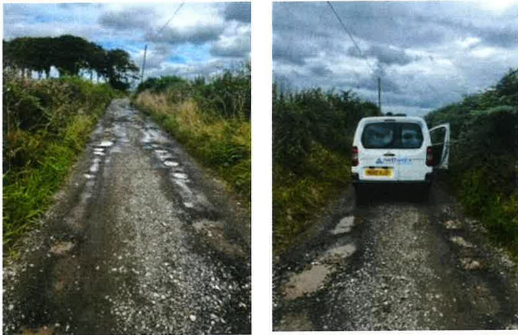
Figure 2: Photographs indicating the width and poor physical condition of the existing lane.
