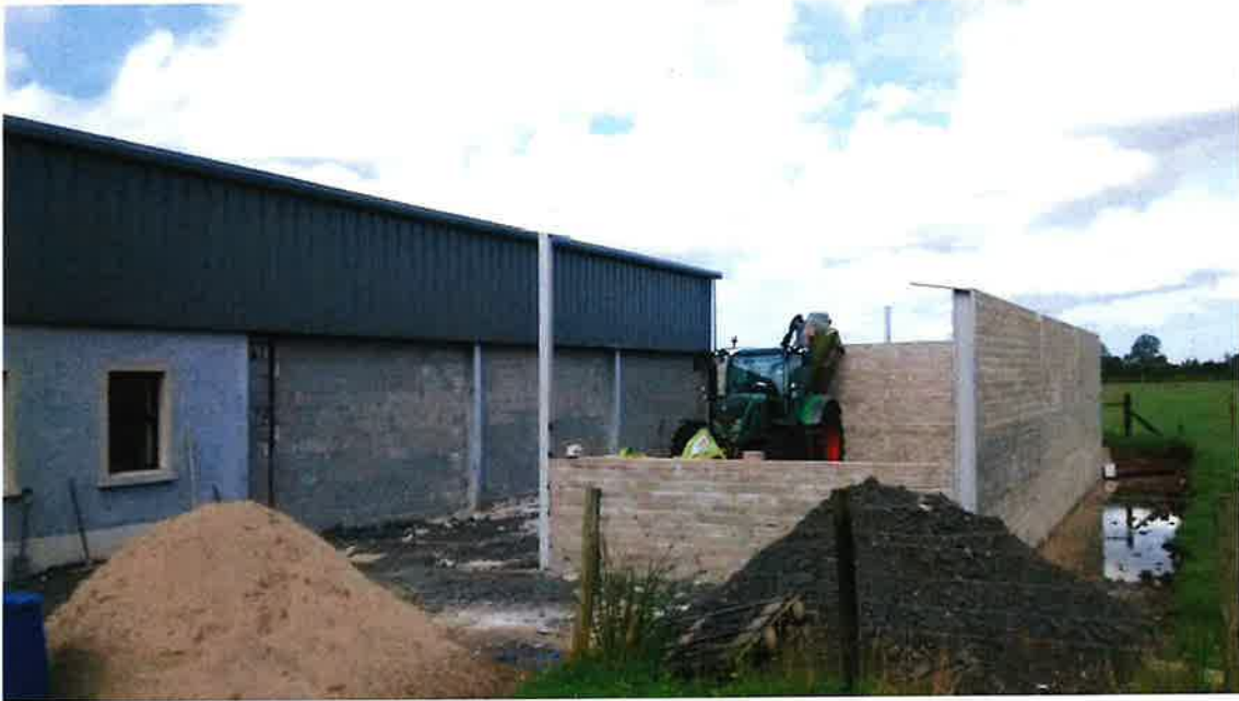
Photograph 4 – August 2015 – Building 3 is under construction. Note, it is self-contained and constructed onto the gable of Building 1 as a single entity and separate building. It's also evident that the render on the gable and the corrugated tin at roof level of Building 1 had to be removed to facilitate the construction of Building 3.
