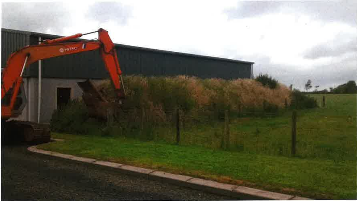
Photograph 1 – July 2015 – Works about to commence the removal of the earth bund in preparation for the construction of Building 3. Note the completed nature of Building 1.
