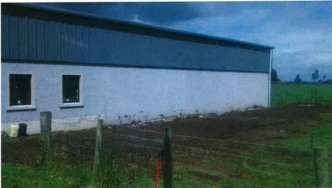
Photograph 2 – July 2015 Earth Bund removed. Note the finished Gable end of Building 1 prior to the construction of Building 3. The gable is completed in corrugated tin sheet with rough rendered walls indicating Building 1 was a distinct building and not part and parcel of an overall larger structure including Building 3.
