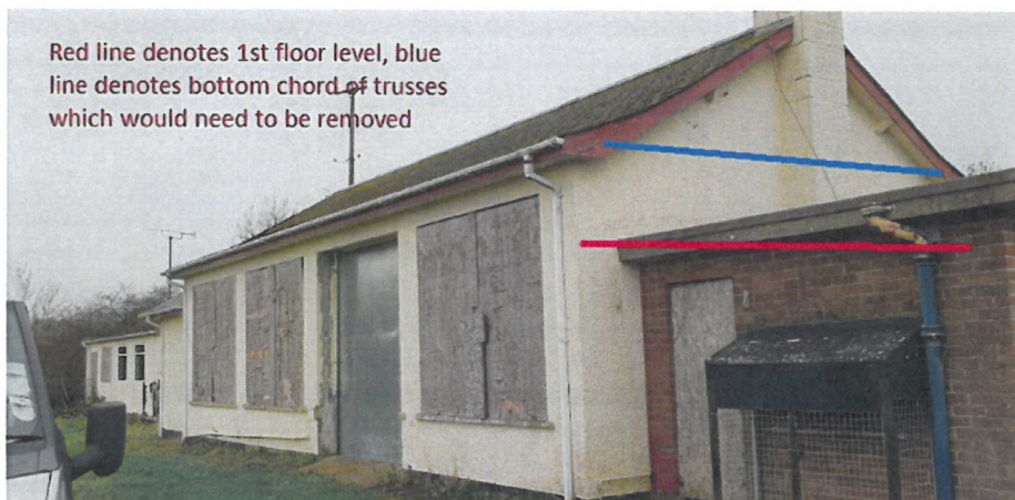
Photo 8 – Illustration of clash between trusses and clear space 1 st floor level
