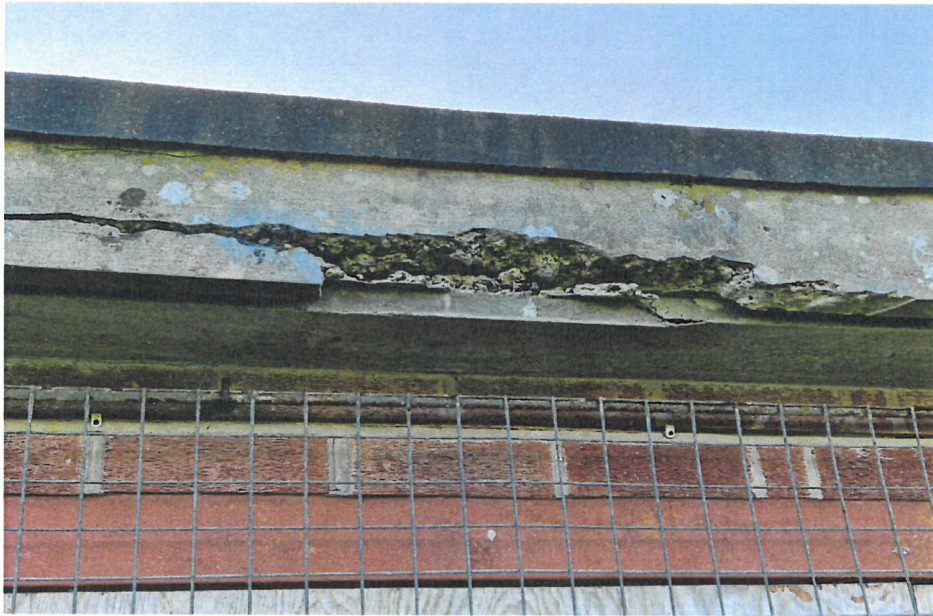
Photo 4 – Spalling of flat roof slab
