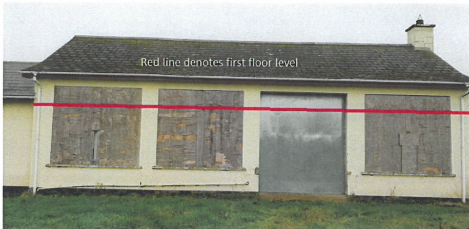
Photo 7 – Illustration of clash between existing windows and 1 st floor level
