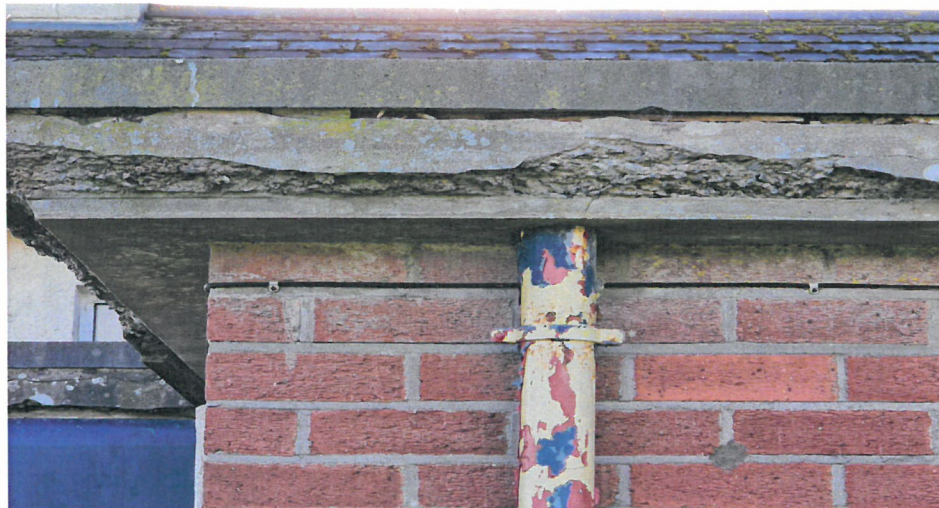
Photo 3 – Spalling of flat roof slab
