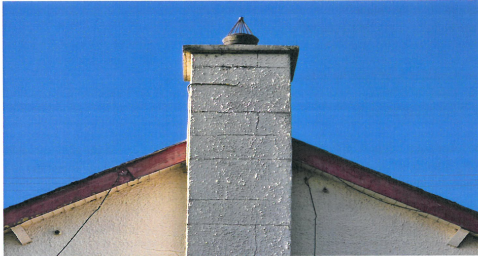
Photo 2 – Cracking at External Chimney
