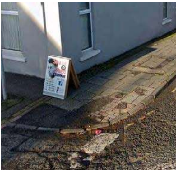
Current Condition - Uneven surfaces and trip hazards.
