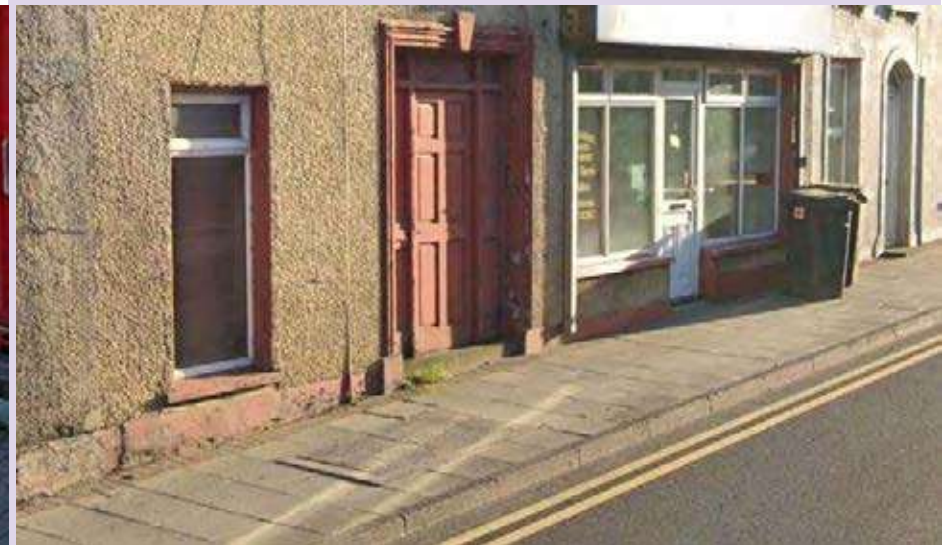
Current Condition trip hazard.
