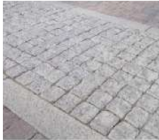
Detail paving to Footpaths at building edge or services: Granite shallow sett
