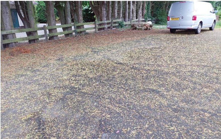
Figure 5. Leylandii root disturbance to tarmac driveway at 43 Semicock Road.
