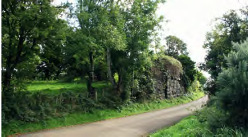
Derelict stone bridge on Hillside Road
