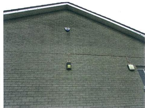
External Emergency Luminaire
