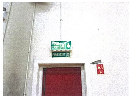
Typical Exit Sign
