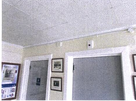
Disabled Alarm Indicator
