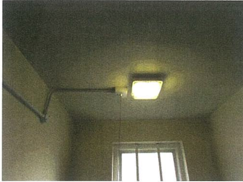
Typical Corridor Lighting
