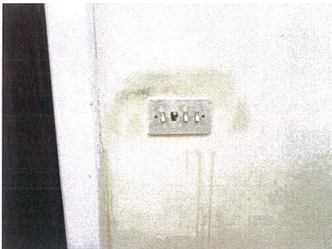
Typical Light Switch
