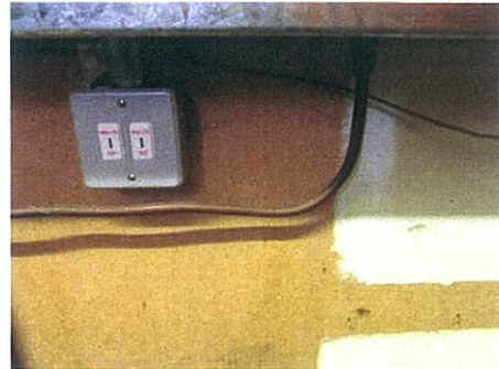
Emergency Lighting Test Switch
