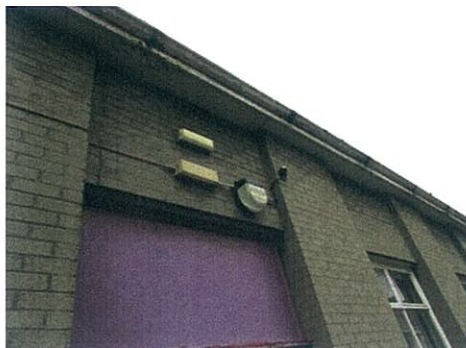
External Emergency Luminaire
