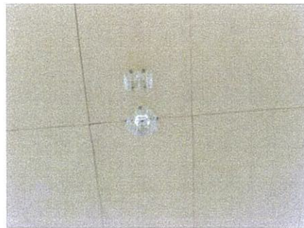
Fire Alarm Source
