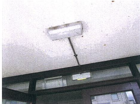
Corridor Emergency Lighting
