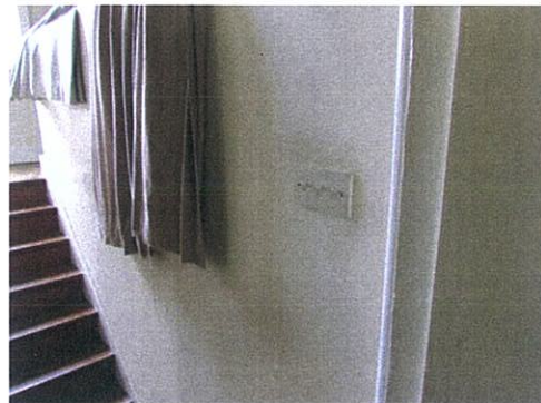
Typical Light Switch
