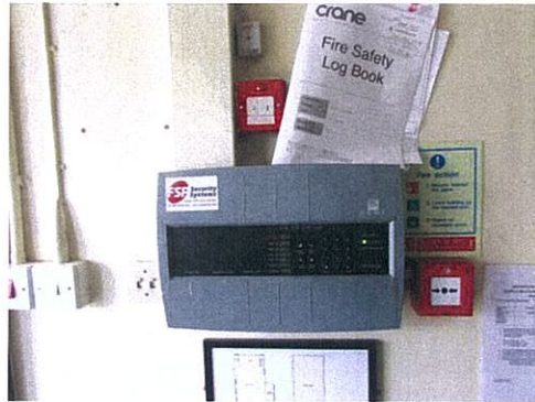
Fire Alarm Panel
